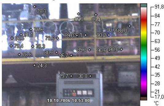
Detail termogramu horkovodu:
